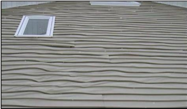
Figure 9. Opposite Wall Distortion
