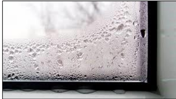
Fig 01-2: Interior Glass Condensation
