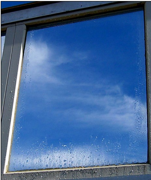
Fig 03: Silicone glazing residue causing picture framing (beading of the water due to silicone residue)
