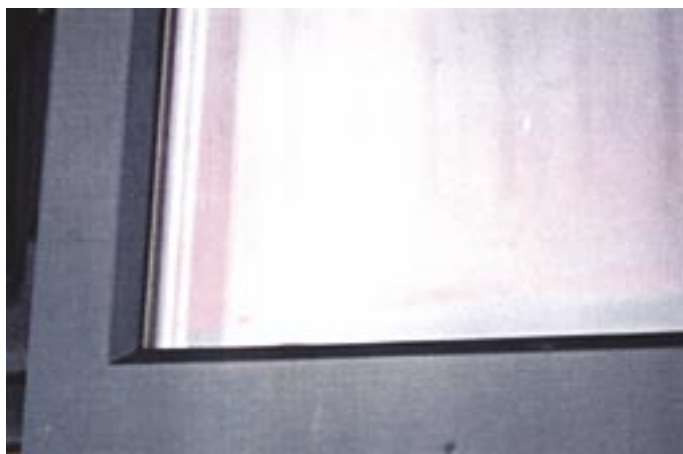
Fig. IG16-2. Photograph showing chemical fogging of low-E IG unit. Solvent vapors on the low-E coating results in a purple color when viewed in reflected light.
