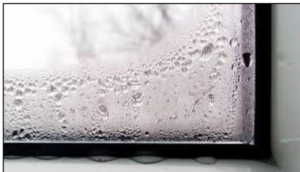
Fig 01-2: Interior Glass Condensation
