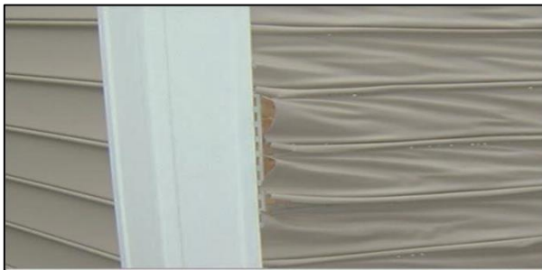
Figure 2. Vinyl Siding Distortion
