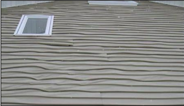
Figure 9. Opposite Wall Distortion
