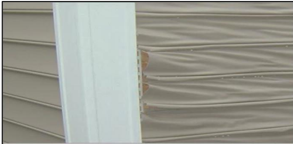
Figure 2. Vinyl Siding Distortion
