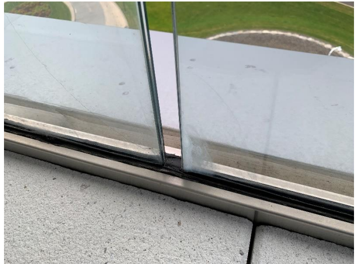
Figure 1. Example of edge defects in laminated glass railings installed in cement-based grout.
